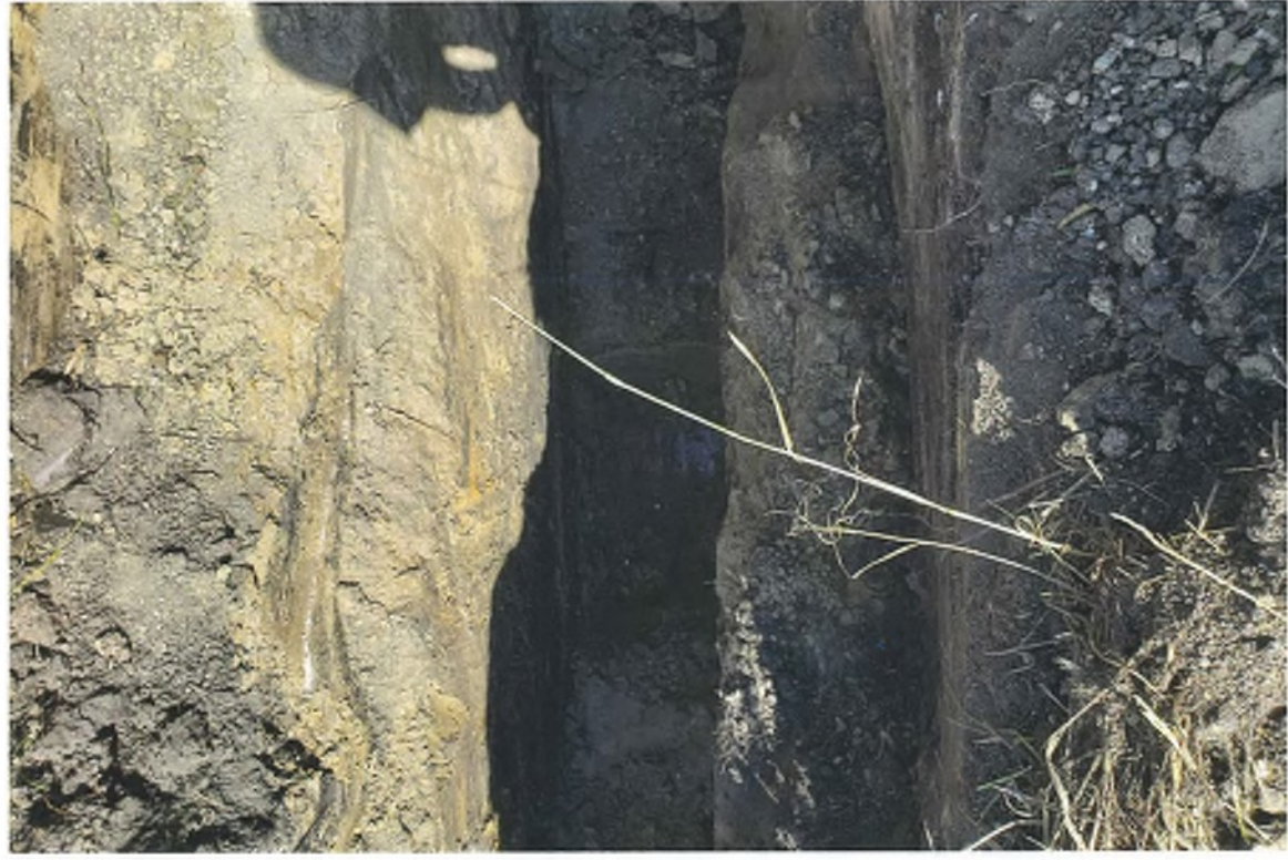
11:39 AM. PICTURE#4 IS LOOKING WEST AT EXPOSED 2.65' O.D. COUNTY TILE GPS# 1092 65 ABOVE TILE 6.86' TO TOP OF TILE (ALSO SEE SKETCH (2 OF 3) FOR DETAILS)
