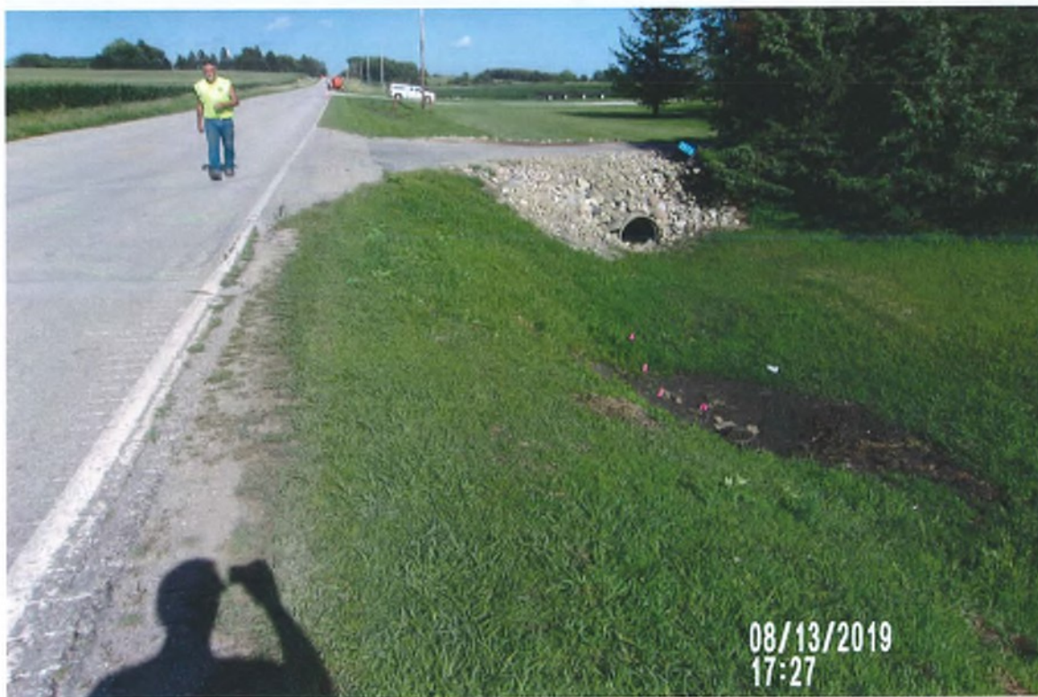
PICTURE # 1186 IS LOOKING WEST TOWARDS WEST DRIVE ENTRANCE FOR 3576 CO HWY D25 SHOWING 18" BEEHIVE INTAKE IN DITCH WITH COUNTY TILE RUNNING E-W
